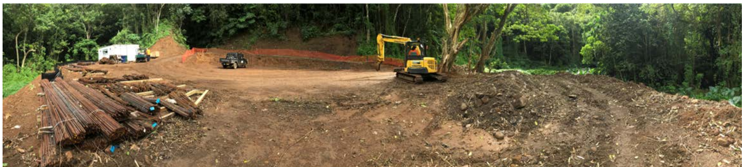
Earthworks underway at the Turangi intake site to prepare for a new water storage tank
