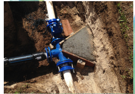
Above: A connection from new Stage1 Ring main into existing sub main feeder line.
